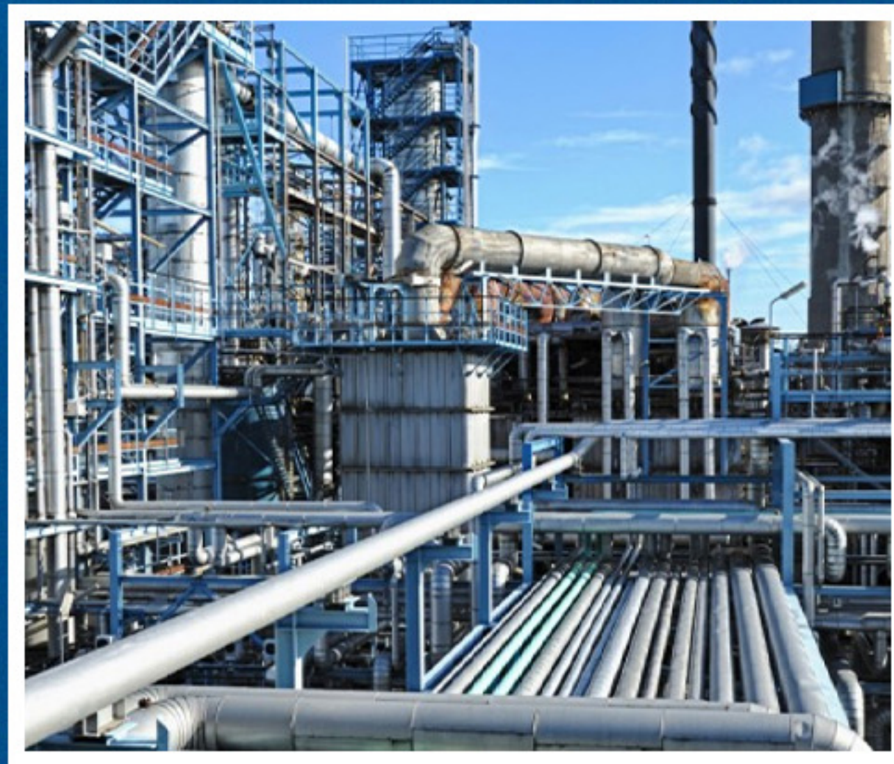
Instrument Air & Membrane Systems
