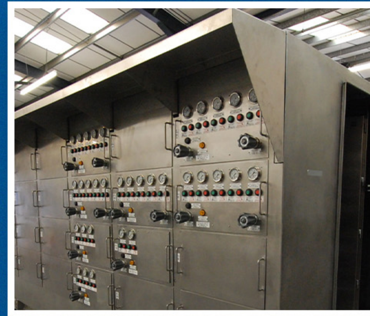
Wellhead Control Systems
